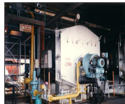
Figure 5 : Mechmar boiler –steaming capacity 20 000 lb/hr at 150psi
